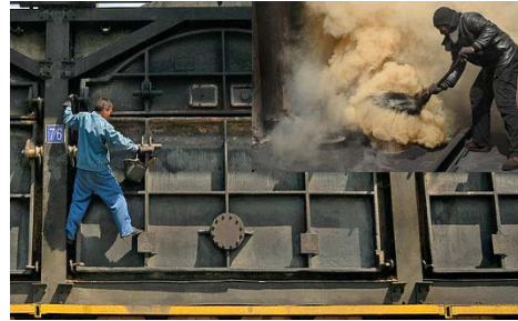
Modern coke ovens
