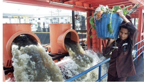
Recovery from wastewater
